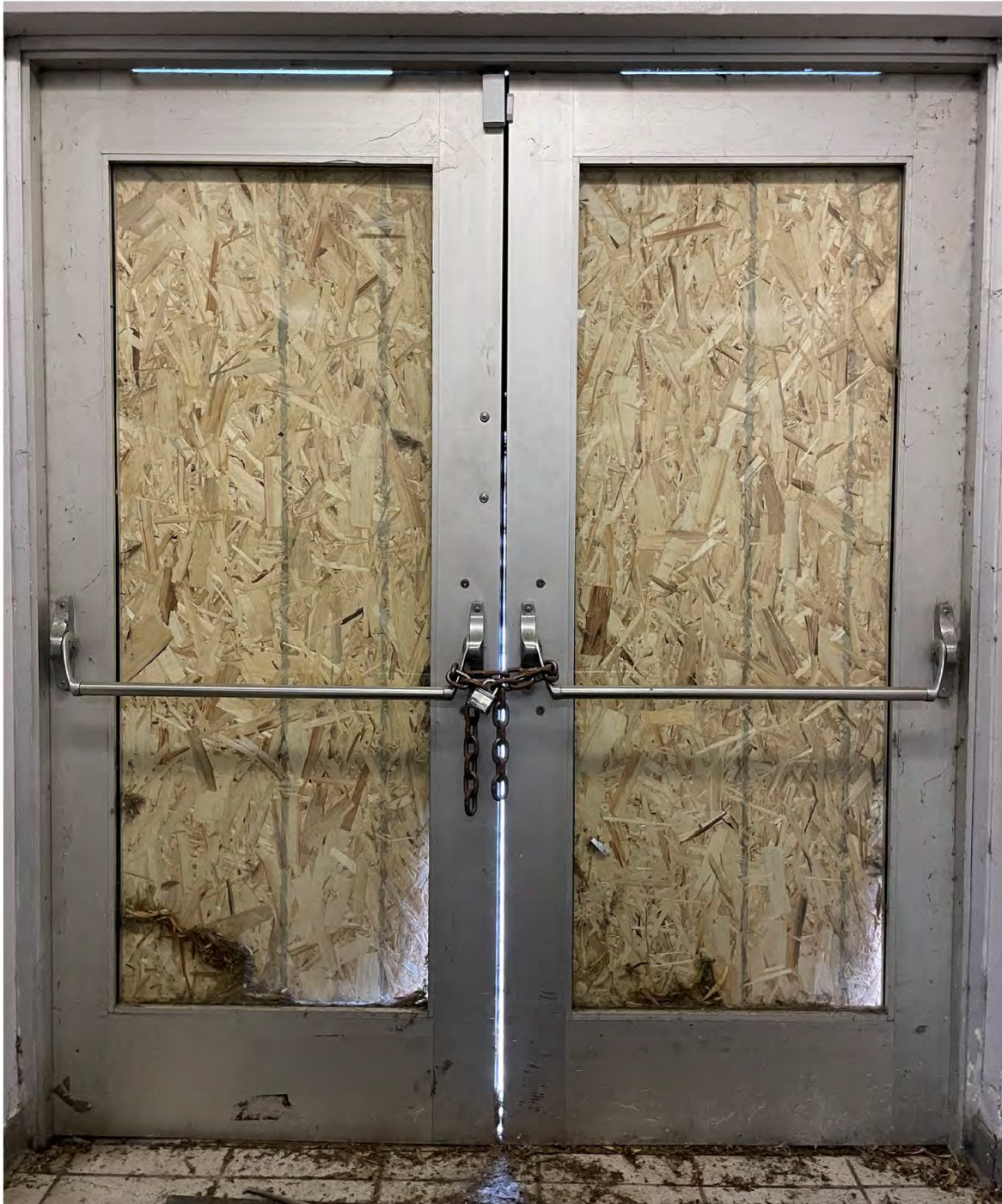
Figure 14. East Wing, framing and hardware of typical entry door (view northeast, from interior hallway, east wing). Image: Nina Fresco, 2023
