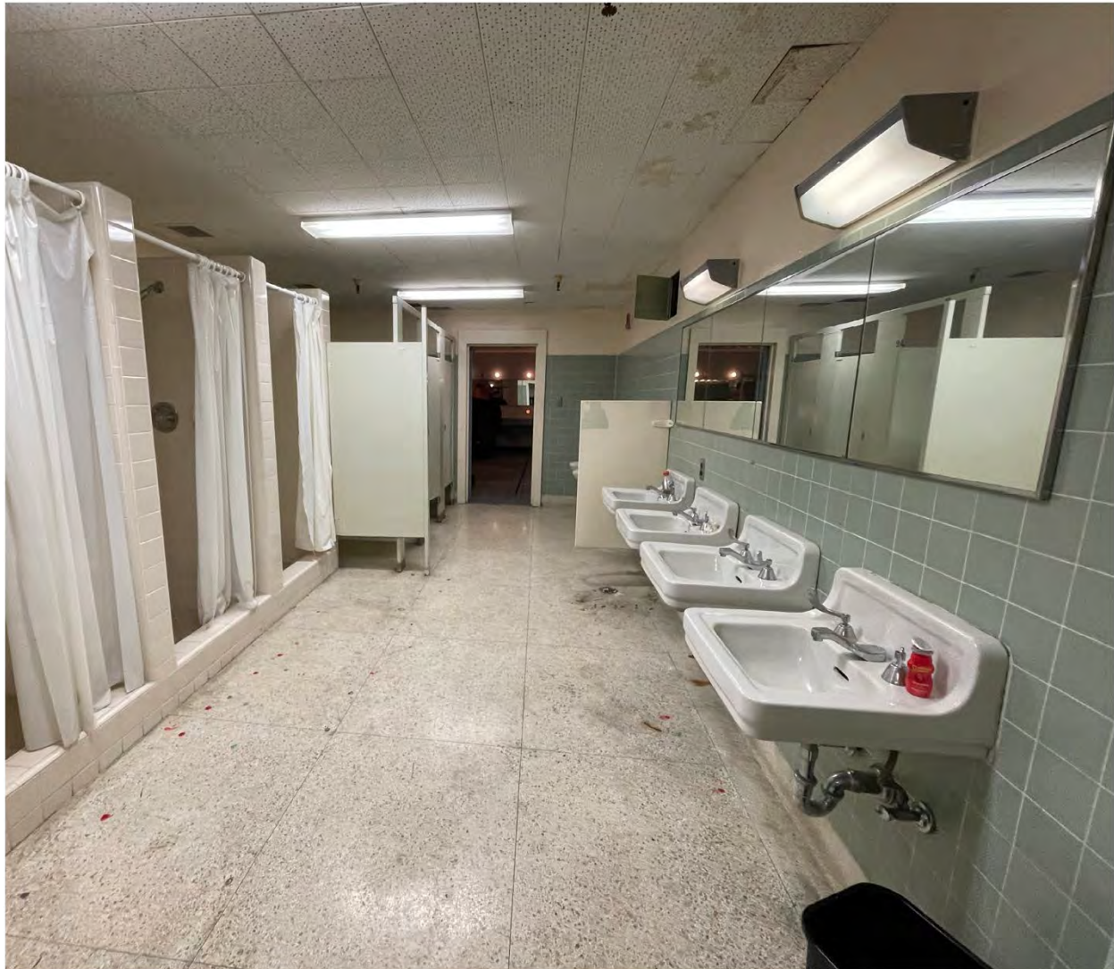
Figure 30. Dressing room, original bathroom tile and fixtures (view northwest). Image: Nina Fresco, 2023
